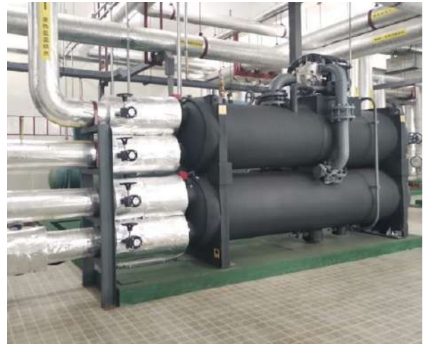
Waste Heat Recovery System in Tianjin Data Center
