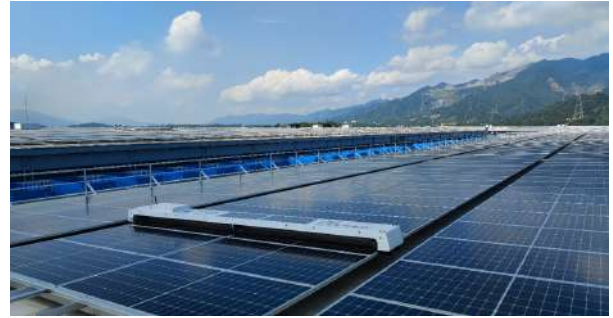
Tencent Data Center Roof Photovoltaic
